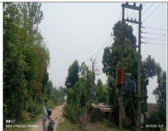
5. Transformer (point source)
