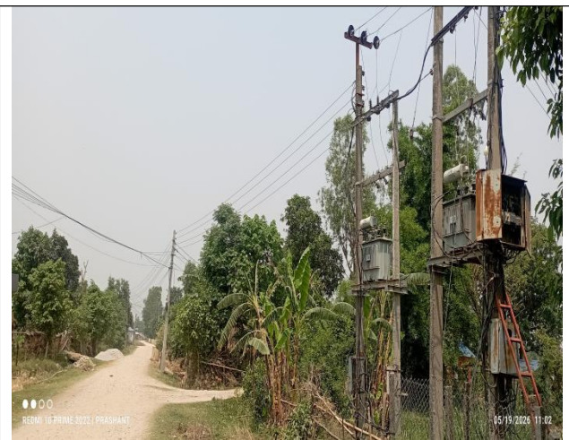
8. Transformer ( point source)
