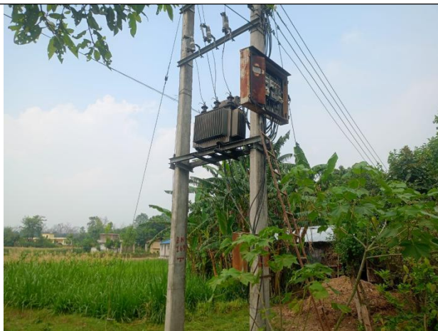
9. Transfoemer at Lamichhane Tole ( Paal Bazar)
